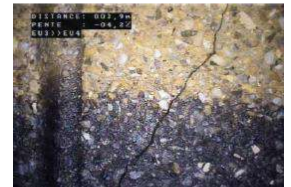
Rue Louis Pergaud (fissure)
